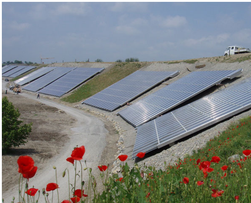
Fig. 2.2.11. On a slope (Schüco), Crailsheim, Germany (by Stadtwerke Crailsheim GMBH) [7]. Notice the size compared to the car on top and the man in the background.
