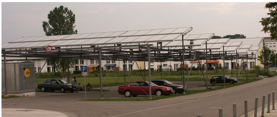
Fig. 2.5.2. Solar collector field "carport" in Neckarsulm (DE). (Source: Solites)
