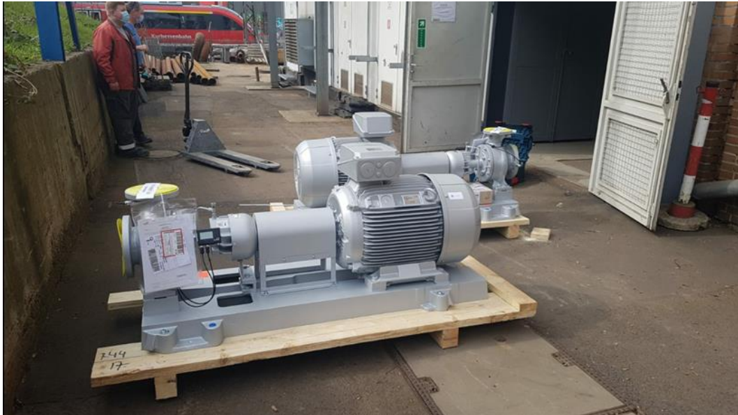
Figure 7: New highly efficient main grid pumps arrived in Marburg
