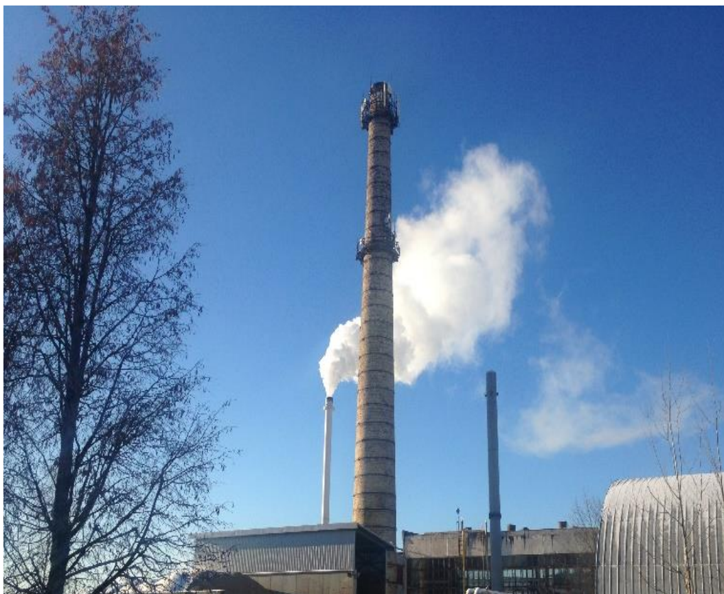
Figure 10: Heat generators in Salcininkai
