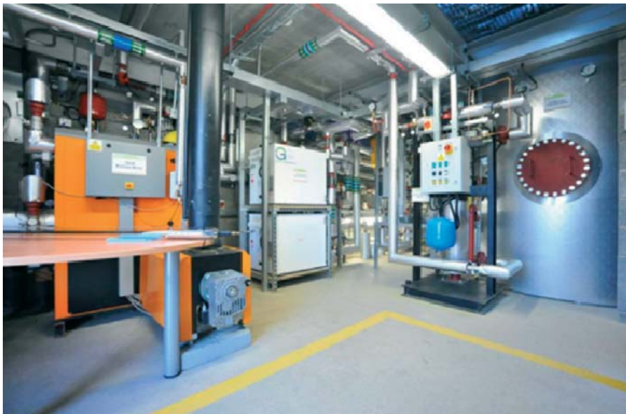
Figure 20: Inside the plant room at the Greenwatt Way system
