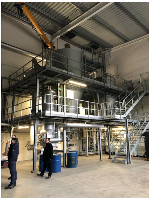
© Fa. Syncraft, Holzvergasungsanlage 400 kW in Emsdetten
